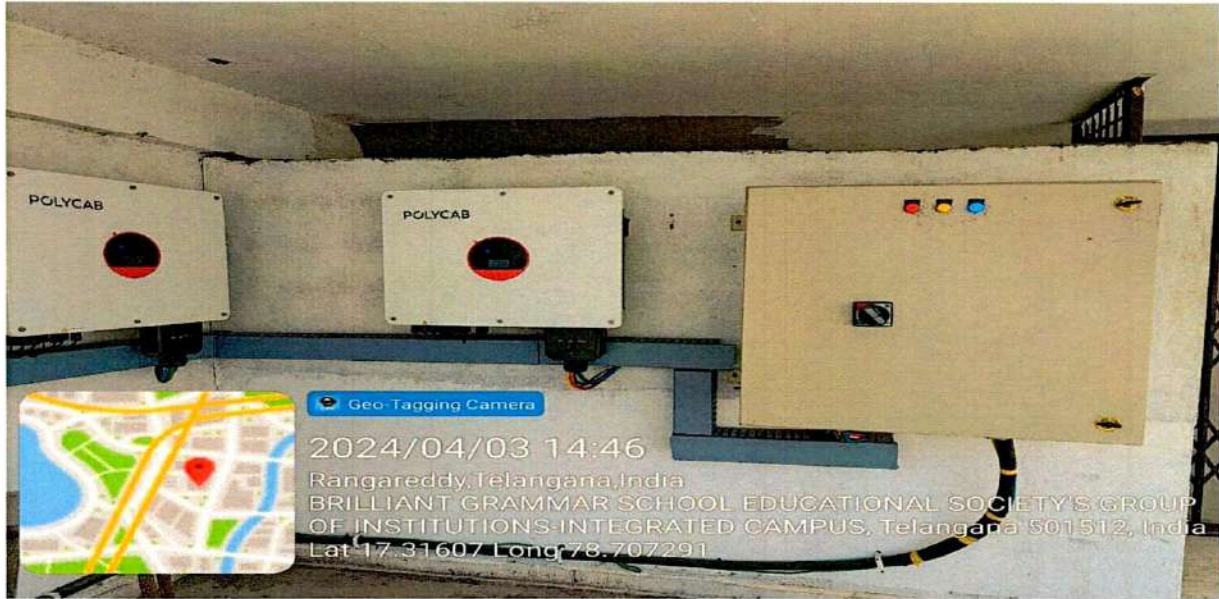
Wheeling to GRID connection.
