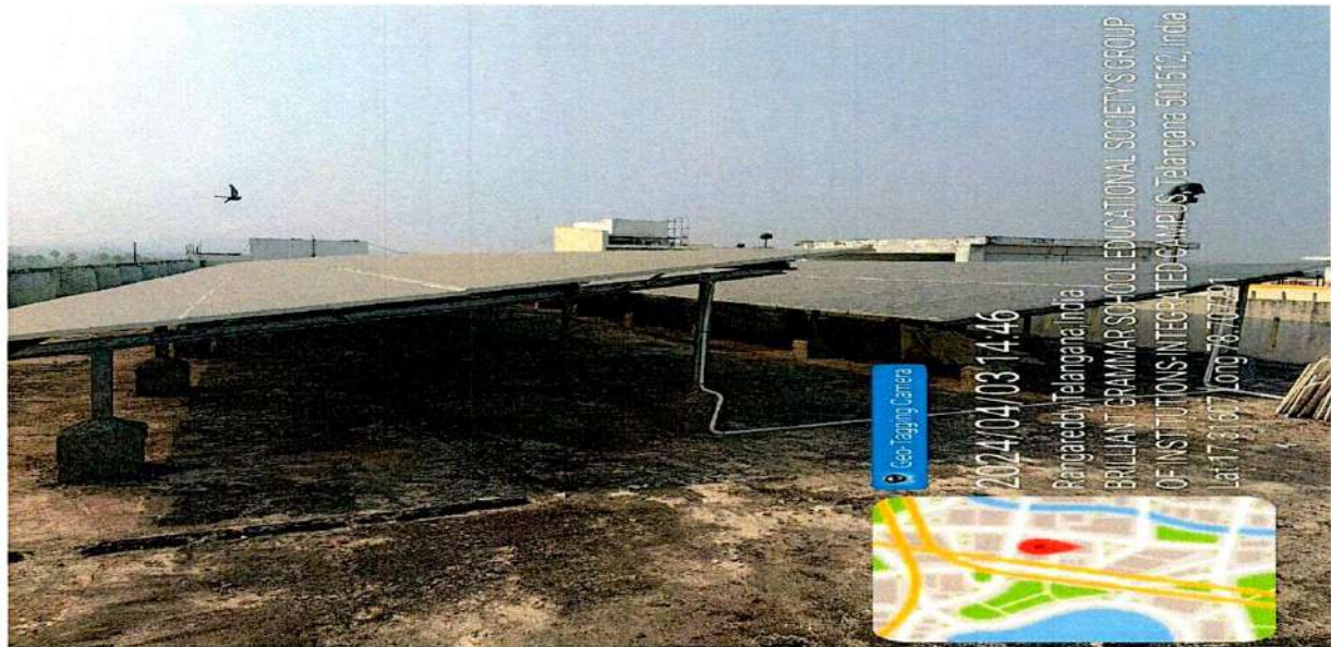
View of Solar Power plant 75 KWP.
